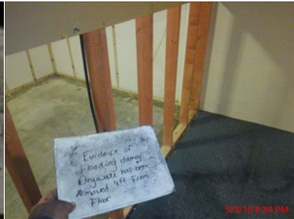
Photo showing inspector's note that there is evidence of flooding damage and that drywall has been removed 4 feet from the floor.
