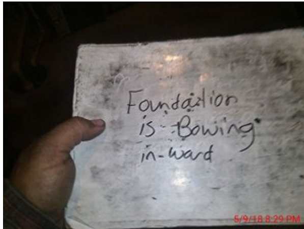
Photo showing inspector's note that the foundation is bowing inward.
