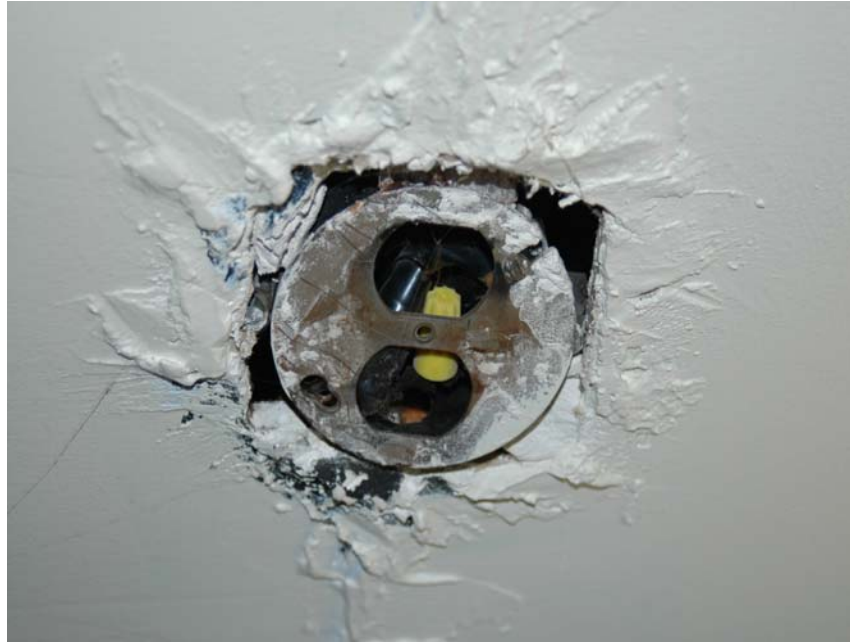
3837 Maryland: Exposed wires in basement junction box.
