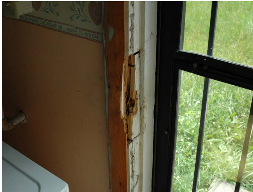
4940 Carolina Street: Broken door jam on the locking side of door with missing strike plate.
