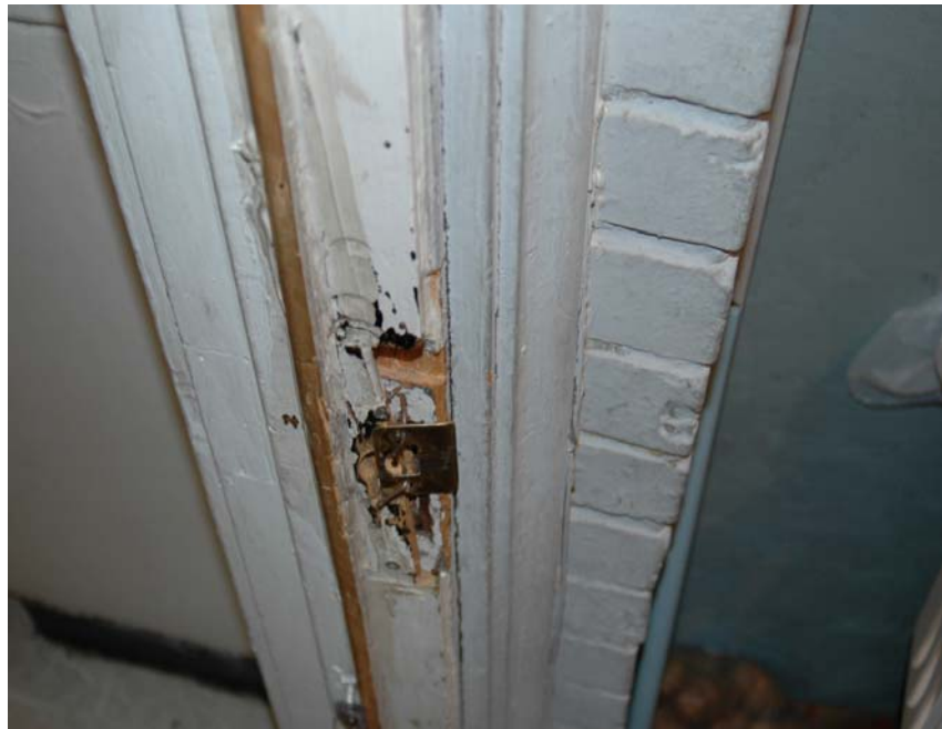
843 Harrison Street: Broken door jam and loose strike plate.
