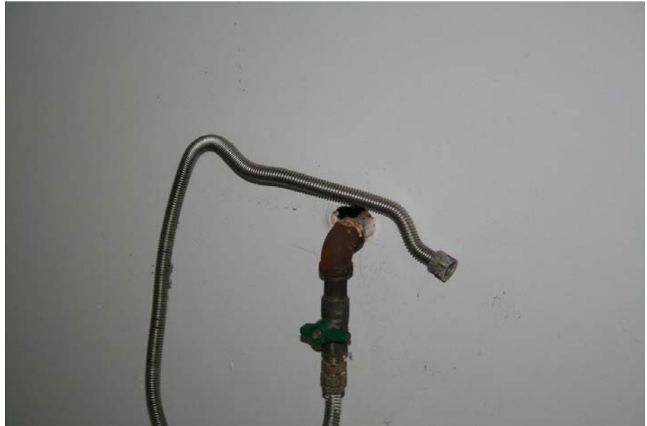
Unit 10: Uncapped gas line
