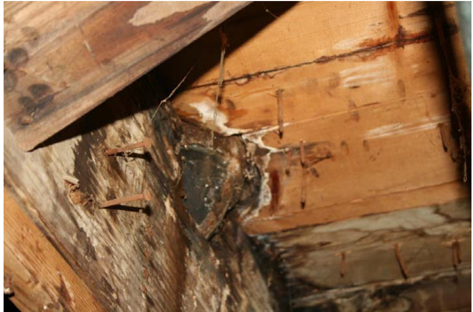
Unit 75: Active water leak from toilet
