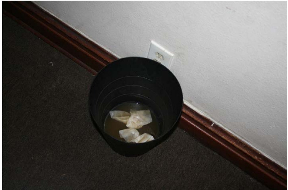
Unit 33: Bucket to collect water from active leak pictured above
