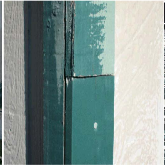
Repairs were made, but the seams were not caulked, and the painting was not completed.
