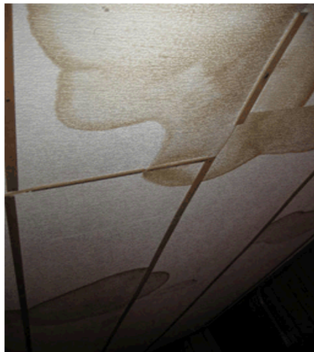
The ceiling tiles showed significant water damage but had not been replaced.
