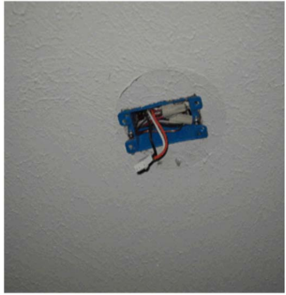
A hard-wired smoke detector was missing, leaving exposed electrical wires.
