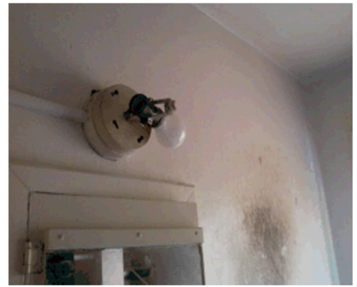
There were missing light fixtures in several of the units. In addition, some of the bathroom fans did not work.
