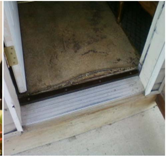
The vinyl was peeling, and the floor was filthy.
