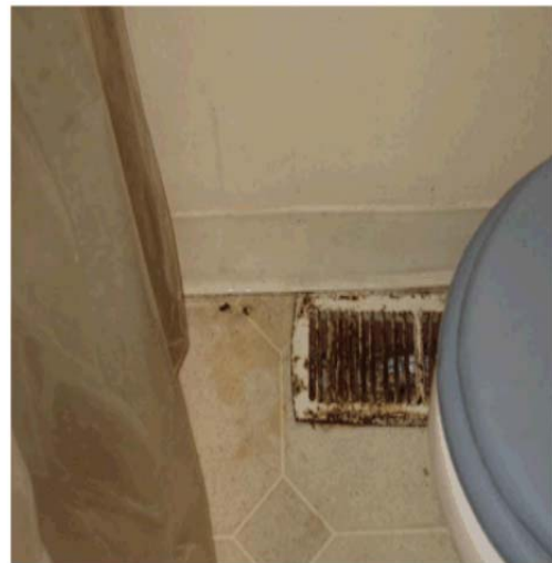
The heating vent was extremely rusted but had not been replaced.
