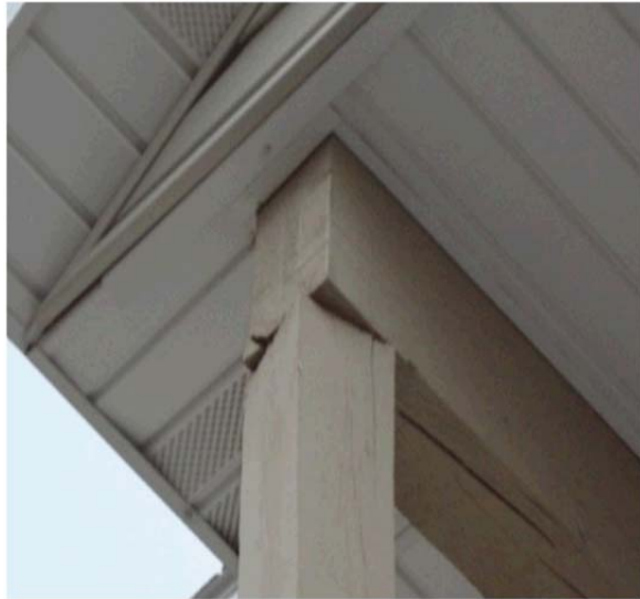
A deck post was severely twisted.
