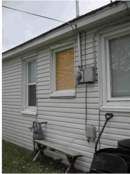
The window was removed, but the siding was not repaired.
