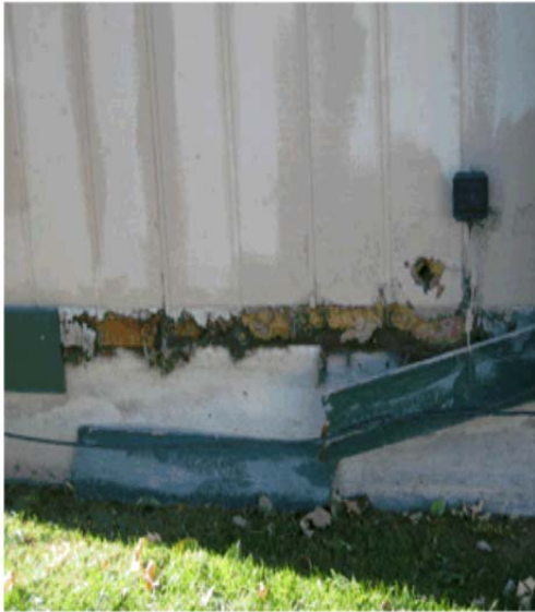
Some of the trim was coming off due to the deteriorated siding.
