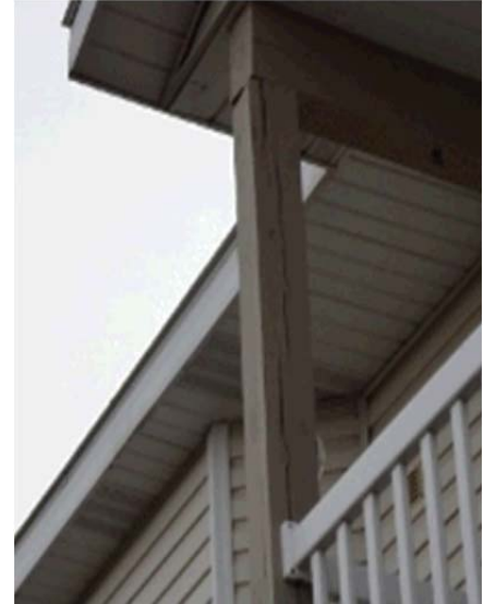
Another deck post was cracked where the railing was attached.
