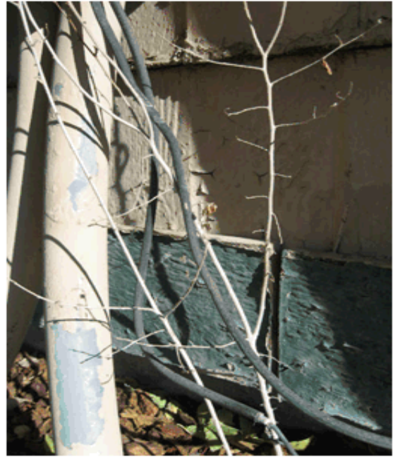
There was no caulk between gaps in the trim, and the paint was peeling.
