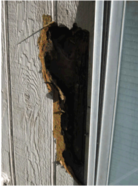
The siding had large holes in it.
