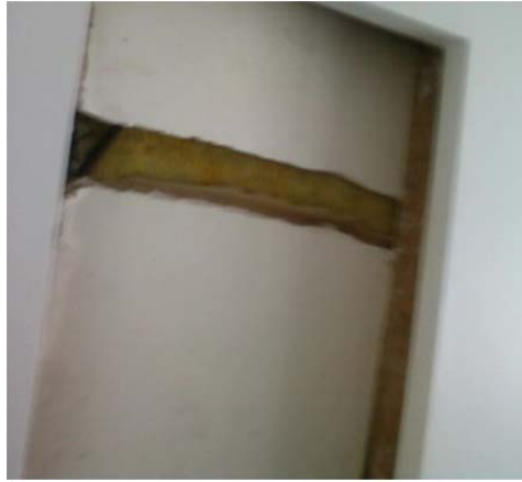
The attic access cover was broken in several of the units, leaving the insulation exposed.
