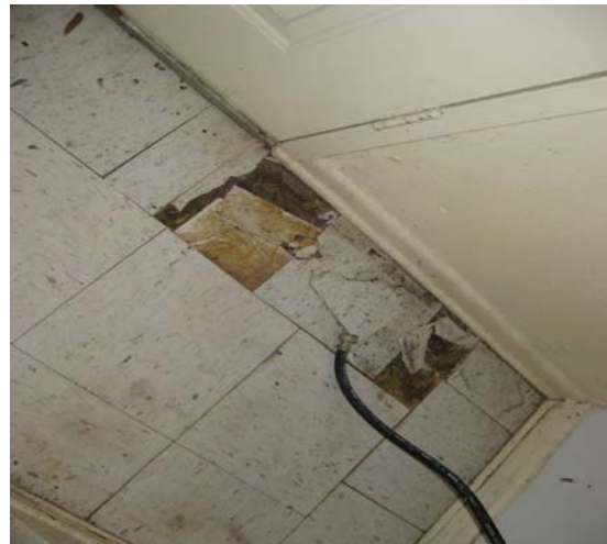
Figure 4: Damaged tile floor – vacant unit
