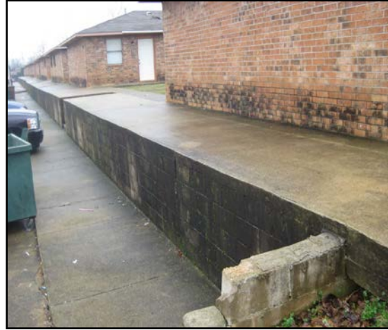
Figure 6: Missing safety railing
