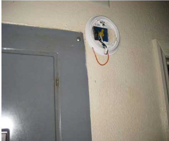
Figure 1: Missing smoke detector -- recently vacated unit
