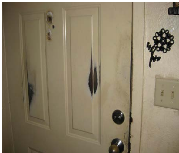
Figure 3: Damaged front door – occupied unit
