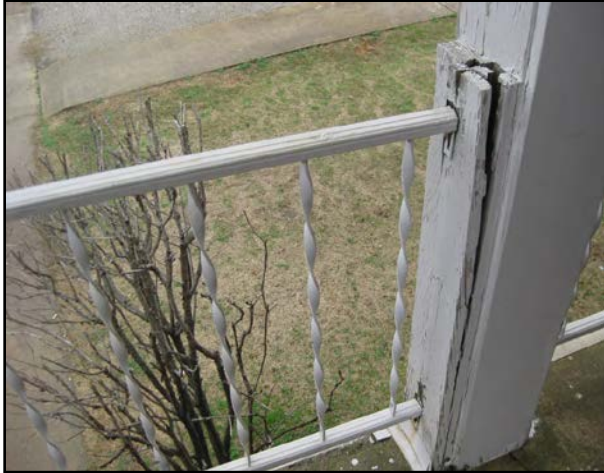
Figure 5: Unsafe second floor railing
