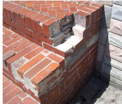
Damaged stairs with no railing
