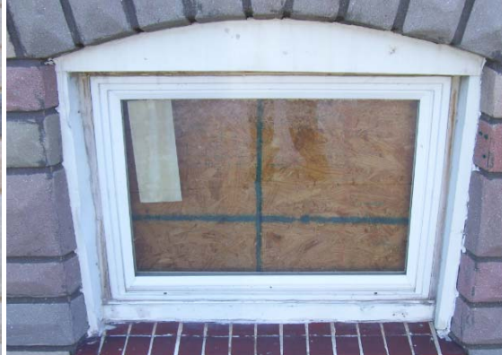
Boarded up egress window
