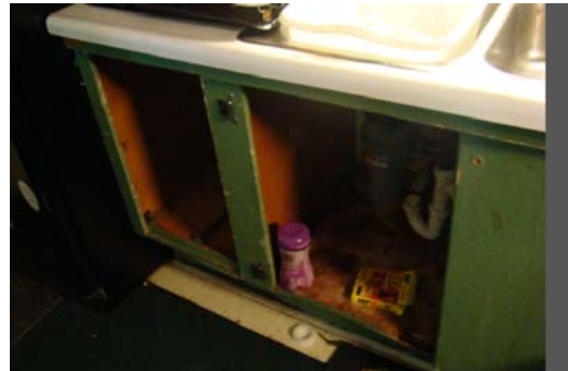
Leaking plumbing and no cabinet doors
