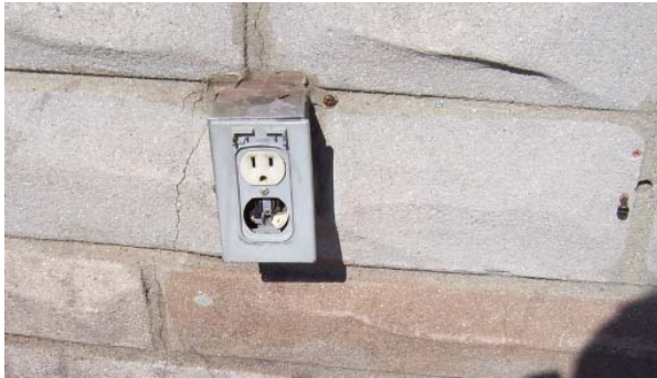
Broken exposed external wirings
