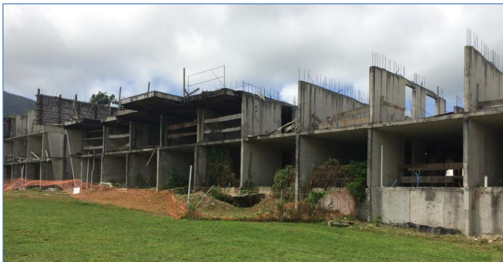
The picture above shows that the housing project site was abandoned and construction was substantially deteriorated.
