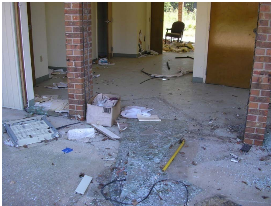
Horton Gardens – Doors and windows missing from the former administration building
