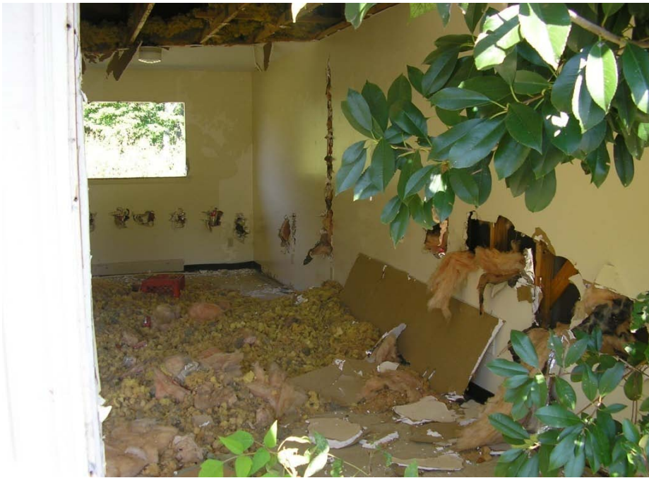
Horton Gardens – Example of unit interior
