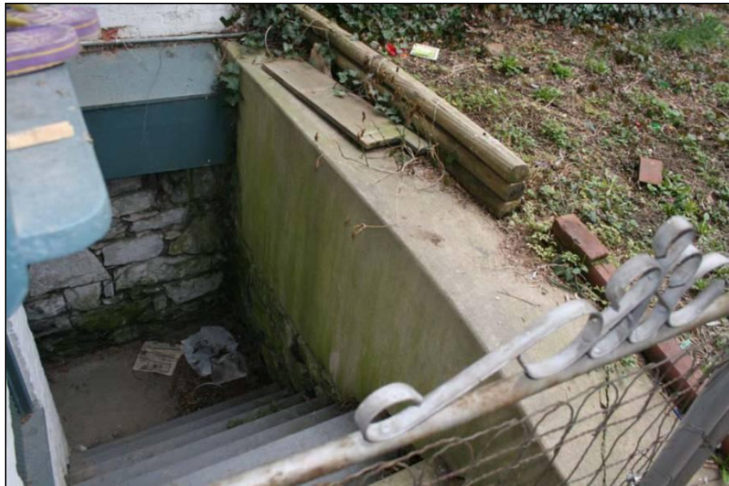
Inspection 7280010: There were a missing handrail and missing railing along the stairs to the basement. These violations were not identified during the Authority’s January 29, 2009, inspection.
