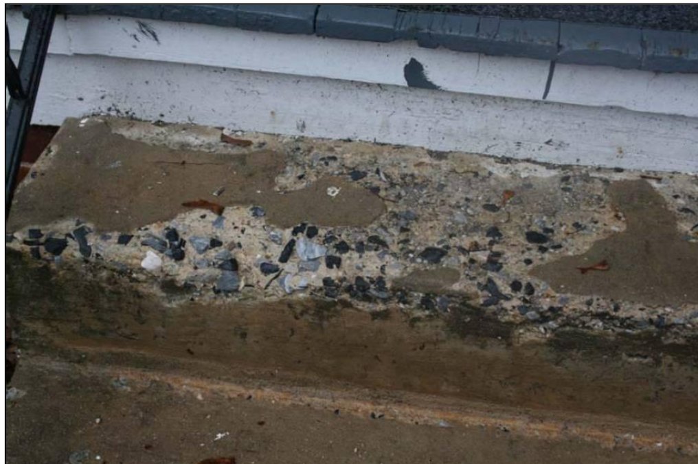
Inspection 7200002: There were damaged cement steps leading to the front door that can cause a tripping hazard. This violation was not identified during the Authority's February 9, 2009, inspection.
