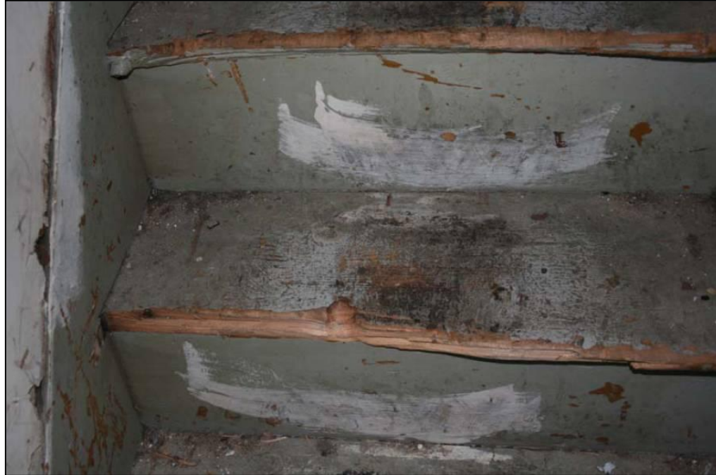
Inspection 3120118: Stair treads leading to the second floor were damaged and can cause a tripping hazard. This violation was not identified during the Authority's January 26, 2009, inspection.
