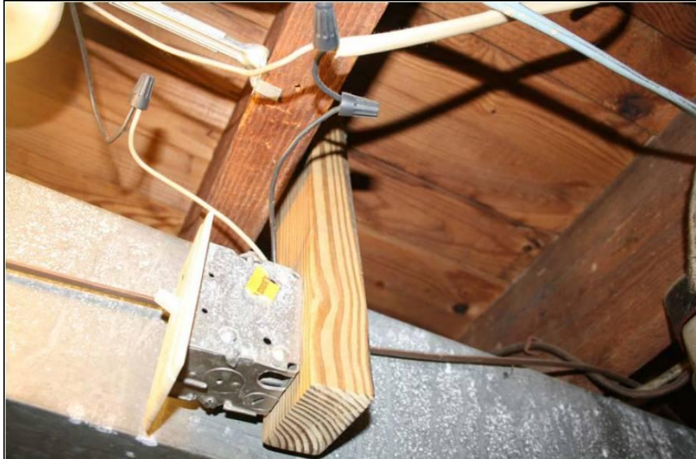
Inspection 7070001: Wire connections were made outside of a junction box. This violation was not identified during the Authority's September 8, 2008, inspection.
