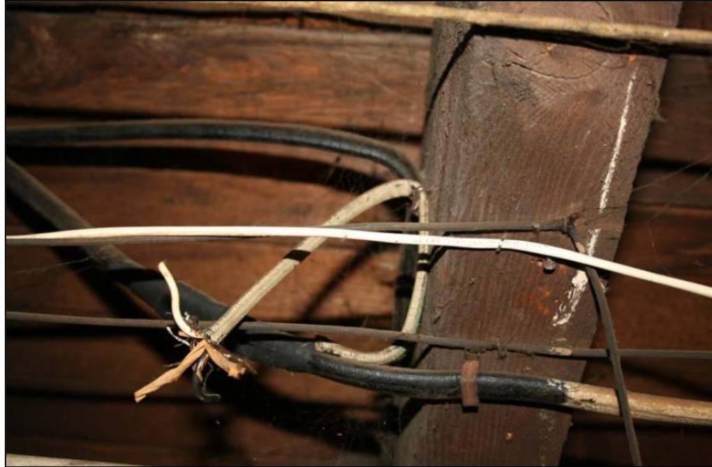
Inspection 7400022: There was an exposed “hot” wire. This violation was not identified during the Authority’s November 6, 2008, inspection.
