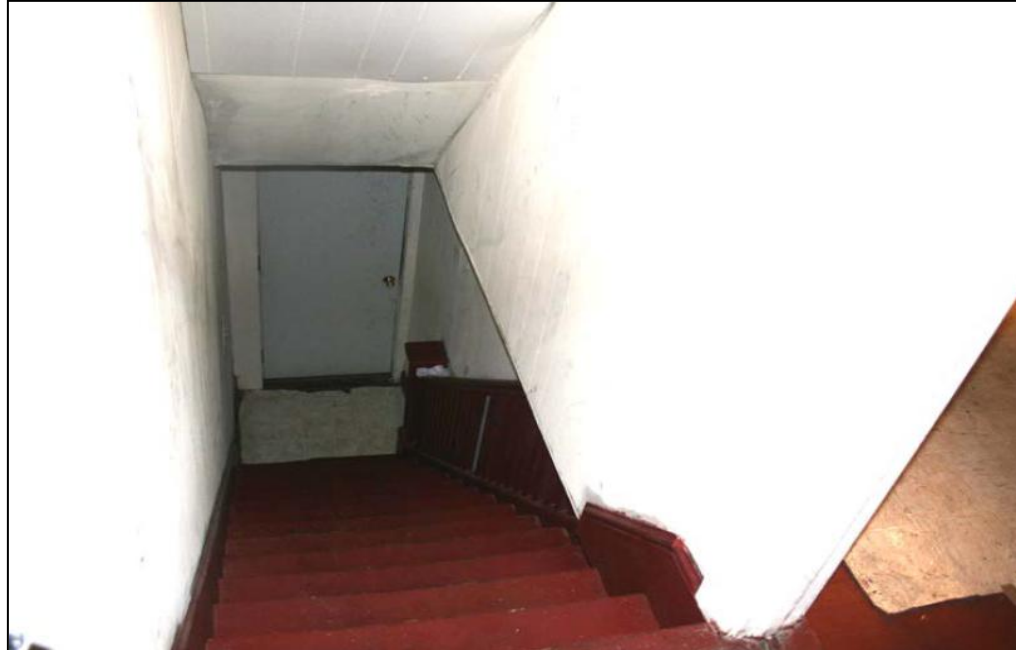
Inspection 3120118: The handrail does not extend the full length of the main stairs to the unit. This violation was not identified during the Authority's January 26, 2009, inspection.
