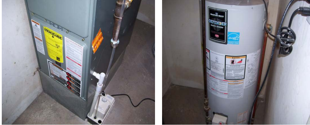
New furnaces (left) and water heaters (right) were replaced in units located at the Windsor Park public housing development.
