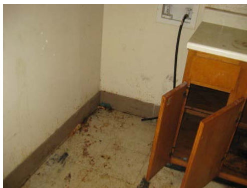
Picture 1: Unit 54. At the time of inspection, this unit had been vacant for more than 3 months. There were slimy substances and food on the walls and floors, flies throughout the unit, a pungent odor, and no visible indication of work having been completed.
