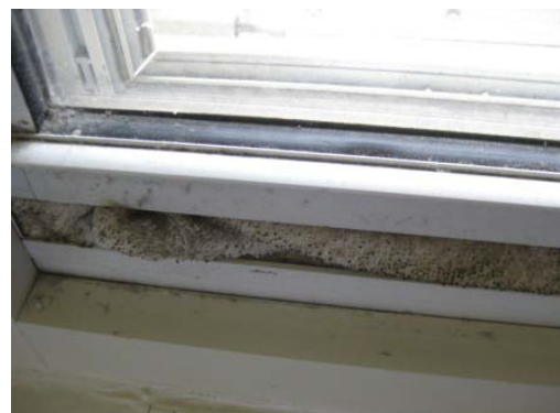
Picture 2: Unit 133. This appeared to be a moldy towel in the window frame. The dirt and chipped paint indicated that the contractor had not cleaned or encapsulated the window frame as required.
