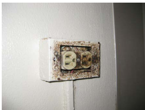
Picture 3: Unit 147. This appeared to be partially painted-over pest excrement.
