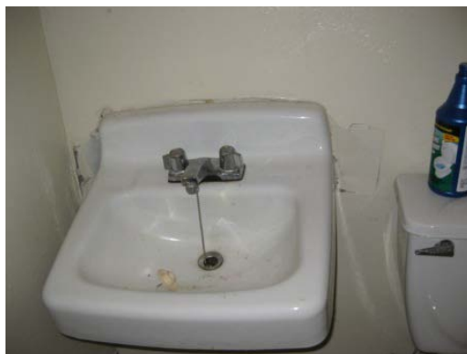
Picture 7: Unit 107. The wall behind this sink was severely damaged. It was unclear who was responsible for the damage.
