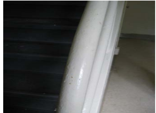
Picture 8: Unit 48. This handrail had paint drippings and rust appeared to have bled through the paint.
