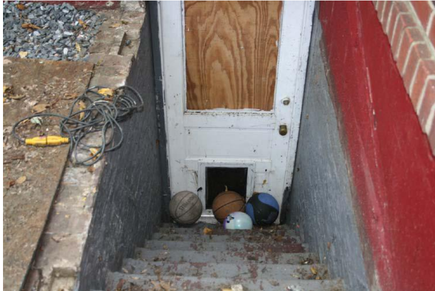
Inspection #7 - There is no railing, no handrail, and no cover over the basement steps. This violation was not identified during the Authority's June 7, 2010, inspection.
