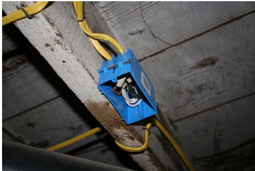
Inspection #10 - The missing junction box cover is a potential shocking hazard. This violation was not identified during the Authority's April 1, 2010, inspection.
