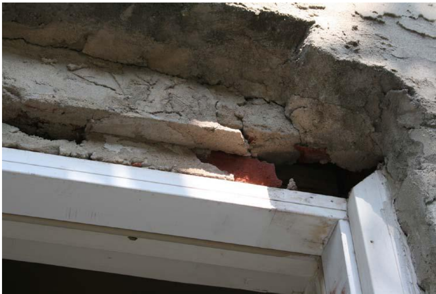
Inspection #14 - There is a hole above the rear door. The hole allows vermin/wind into the wall. This violation was not identified during the Authority's April 28, 2010, inspection.
