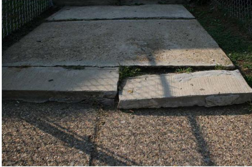
Inspection #18 - The broken concrete walk to the unit is a tripping hazard. This violation was not identified during the Authority's March 2, 2010, inspection.
