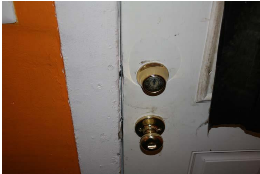
Inspection #16 - The double keyed deadbolt lock poses a trapping hazard. This violation was not identified during the Authority's March 23, 2010, inspection.
